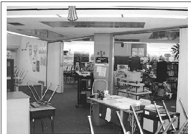
FIGURE 9. Open Plan Classrooms While advantageous for certain teaching methods or student interaction, they have serious drawbacks acoustically. Although partial height partitions or operable partitions eliminate visual distractions, they provide ve
